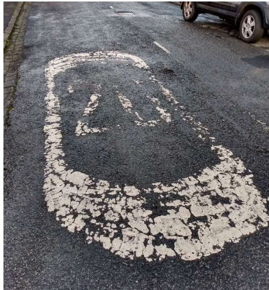
Figure 4 Worn road markings
