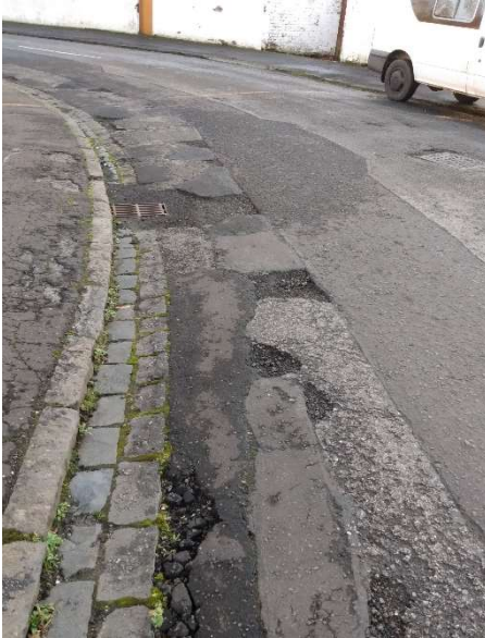
Figure 3 Potholes in the 'riding zone'
